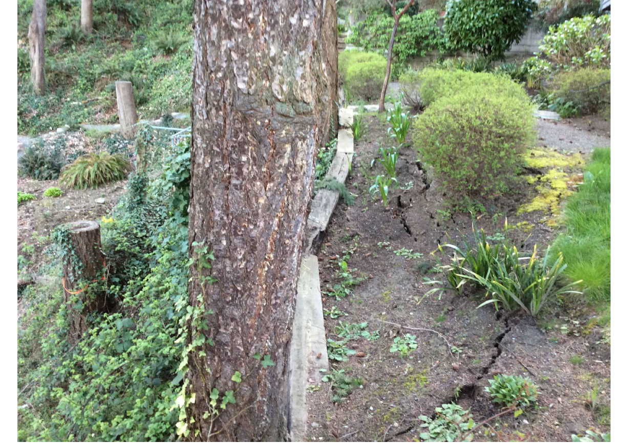
VISIBLE FAILURE OF SLOPE
